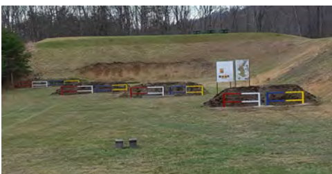
The new turkey and chicken rails were installed and all rails were painted yesterday morning, March 30th. Starting at eight a.m. with Paul Hardy, Mick Malone, Terry Himmler, Jim McCullough, Ron & Marvin Smith and Darren Robinette on the skid steer, we made short work of it.
