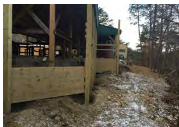
Darren Robinette of Robinette Excavating who worked extensively on this retaining wall project, cut us in a firebreak trail that he used to get equipment in behind the pavilion. Darren used yards and yards of shale from our impact berm walls to lay a trail base.
