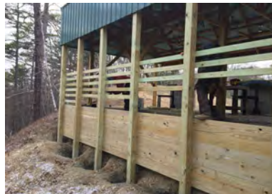
Employees of Frontier Builders working on the retaining wall in February. Owner, Todd Ritchie and his crew did a nice job and will be back in the spring to do the concrete pad under the pavilion in this area.
