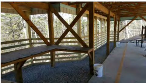
Beautiful work day in February, Darren Robinette of Robinette Excavating, Jim McCullough and Marvin Smith completed the back fill on both sides of the retaining wall. We were glad to get a jump on this project in the winter.
